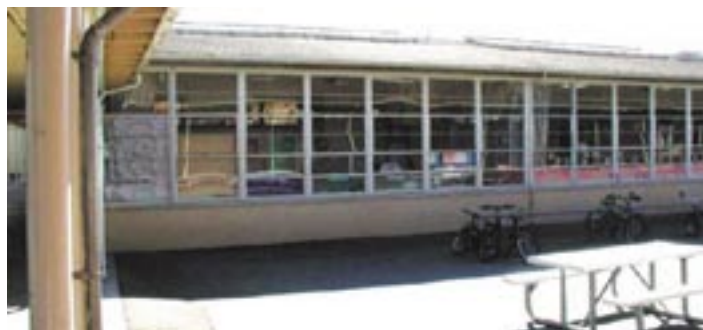
50 year-old wing at Live Oak School: Needs new roof, plumbing, electrical and energy efficiency modifications
