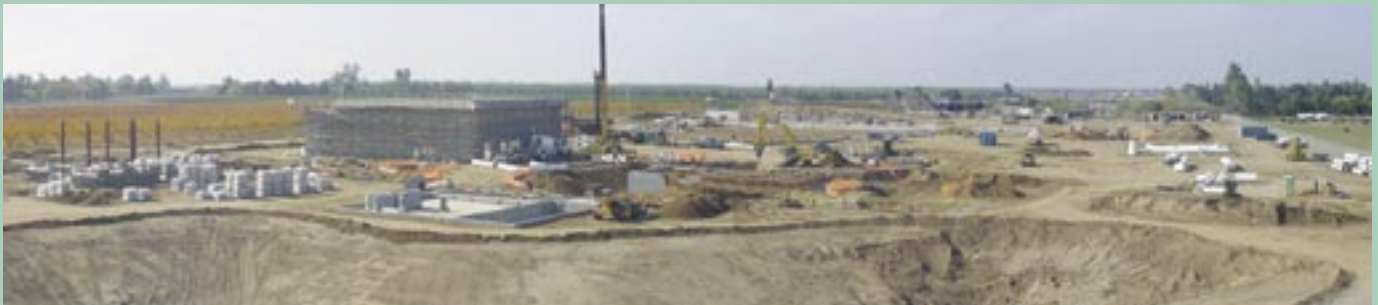
Construction of the new reservoir is underway on Bullard and Leonard Avenues.
